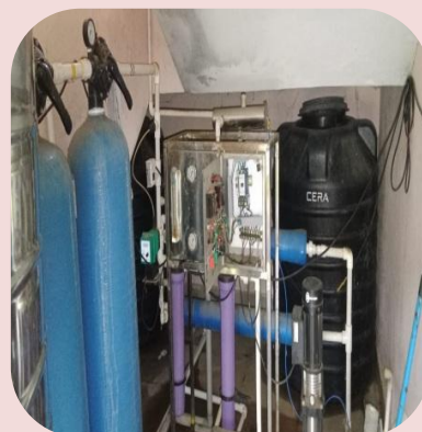
R.O. WATER PLANT
